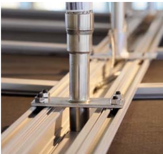
FlexHead sprinkler mounting bracket shown attached to MetalWorks Wings center spine.
