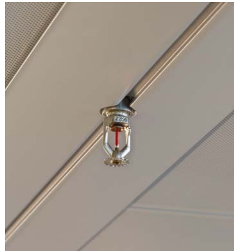
FlexHead sprinkler shown through MetalWorks Wings center spine.
